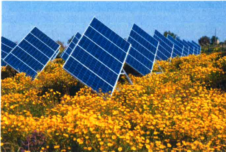
The Chiaramonte Gulfi PV Plant, located in Sicily, is 4 MW in size.
